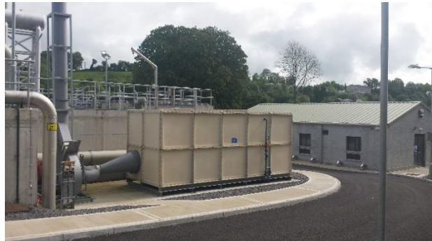
Figure 1 - Monashell OCU in Cavan WWTP, Ireland
