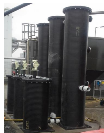
Figure 1 - CrumRubber Pilot Plant
