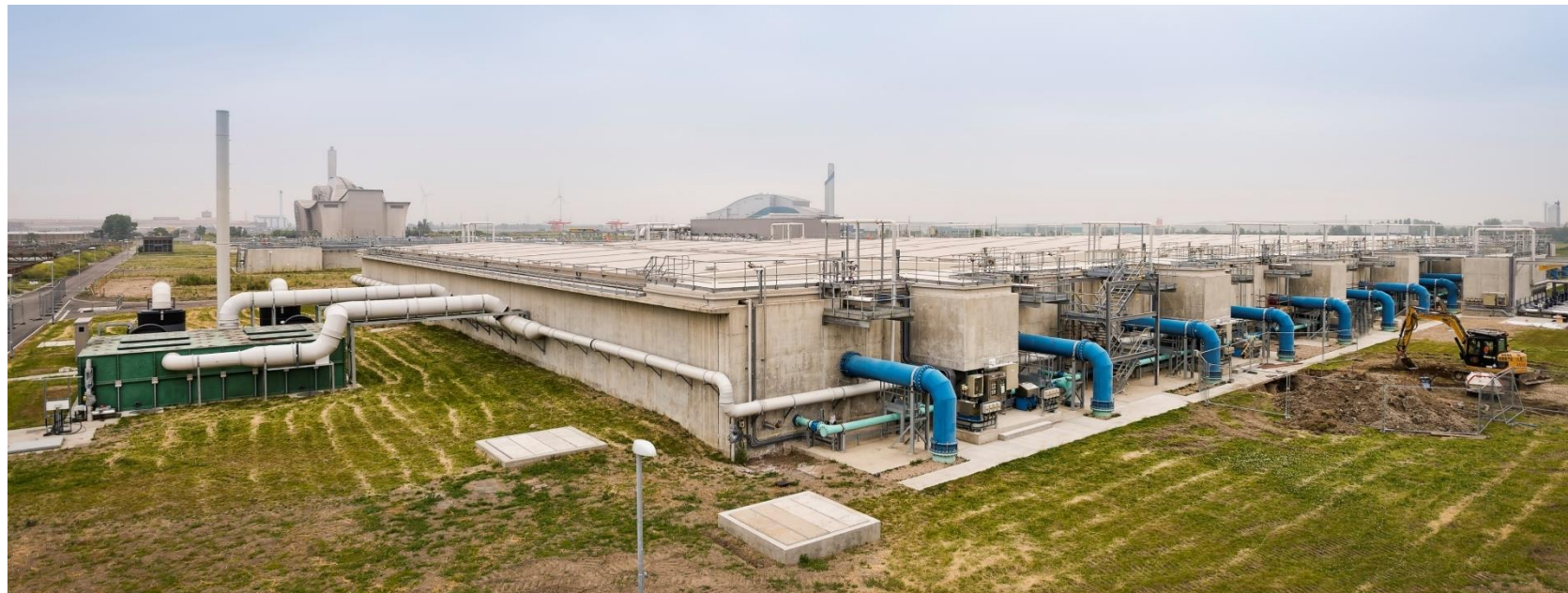
Figure 6 - Mónashell OCU installed in Becton WWTP, London
